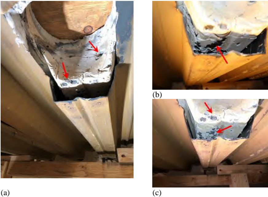
Fig. 4-40. Post-test photographs: (a) slab through-hole used for running a water-cooled loading tube; (b-c) deck delamination from concrete. Localized spalling is indicated by arrows.
